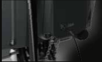
Battery charger on board
